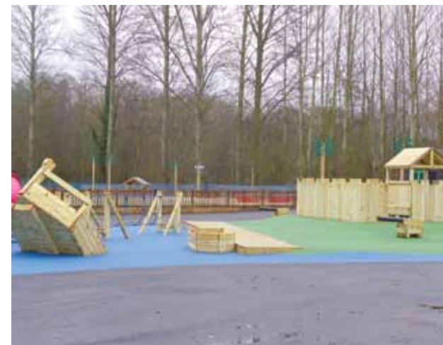
...So a Mega Ship is incorporated with some play trail items to provide access. We also created bespoke "shipwreck" climbing apparatus, a mini fort with cannon for younger users and tied the whole thing together with a jetty, rowing boat and clever use of wet pour colours to provide "land" and "sea."
