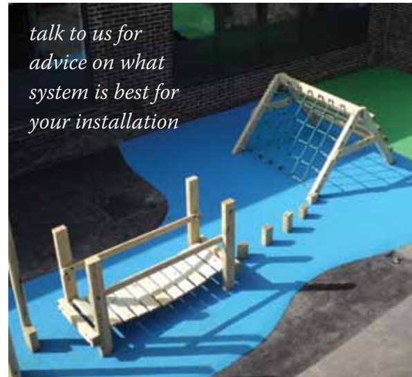
Wet pour in a school playground. Note the use of different colours.
