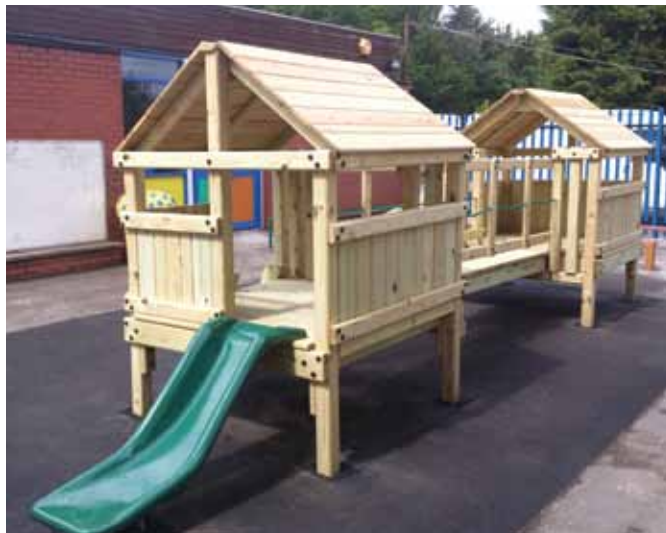
We installed this on an existing wet pour surface (note the patches around the posts). Here the deck height is reduced down to 600mm for a Reception class.
